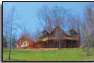
MARS HILL: New home under construction with gorgeous mountain views. A 21' towering, 8" tongue and groove ceiling, hickory kitchen with granite tops. Hand hewed log siding. $525,900 MLS# 410563
